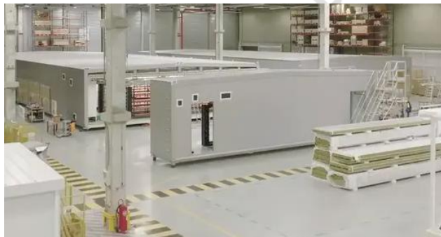
Fotografía 3: Schneider Electric C EcoStruxure™ Data Center Solutions, https://www.se.com/es/es/work/solutions/data-centers-and-networks/modular-data-center/
